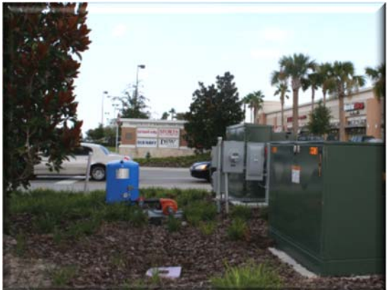
Ground vaults at project entrances should be properly screened.
