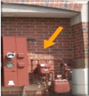
Utility equipment is painted to blend with the building.
